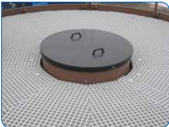
LUIK IN AFDEKKING OP LAVAFILTER
